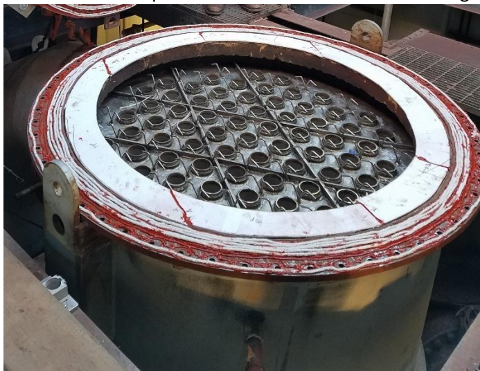
Figure 5. Primary heat exchanger
